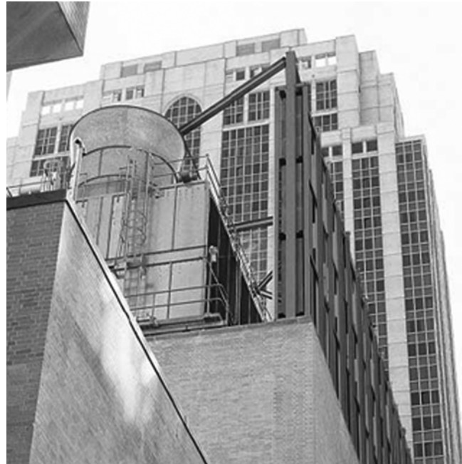
Fig. 1 Cooling Tower Noise Barrier (Courtesy Neil Moiseev)
